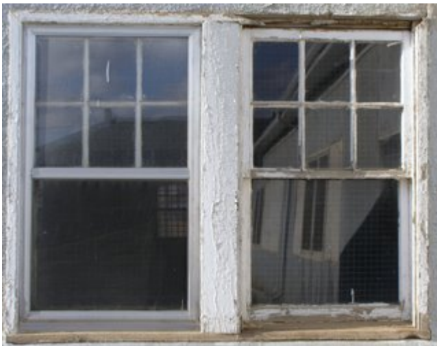
Figure 5 - Flaking Paint on old windows
